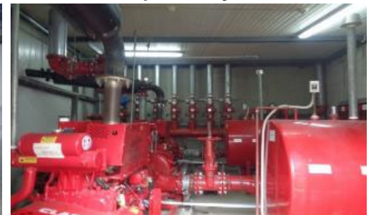
ESFR (Early Suppression Fast Response) Fire Sprinkler Systems
